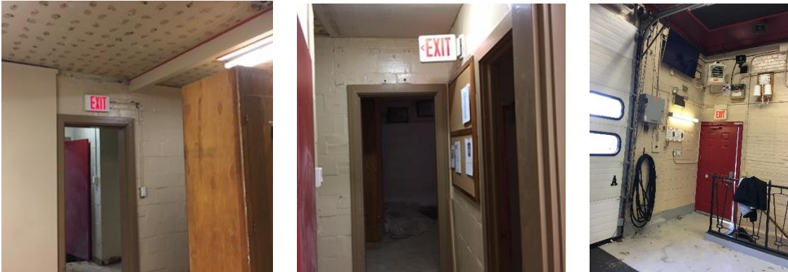
Installed exit signs. Note rooms have no space signage.
