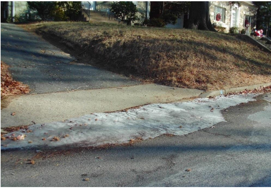
Accumulated ice in the gutter
